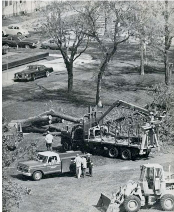
Figure 2: Renovation work on Murphy Square. Reprinted from the Augsburg Echo , September 30, 1977, pg. 1.
